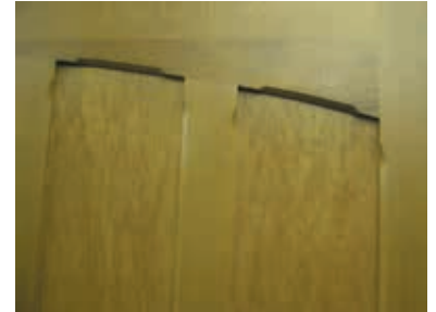
Panel detail of plywood panelled doors with cedar facings showing stopped chamfer profile
